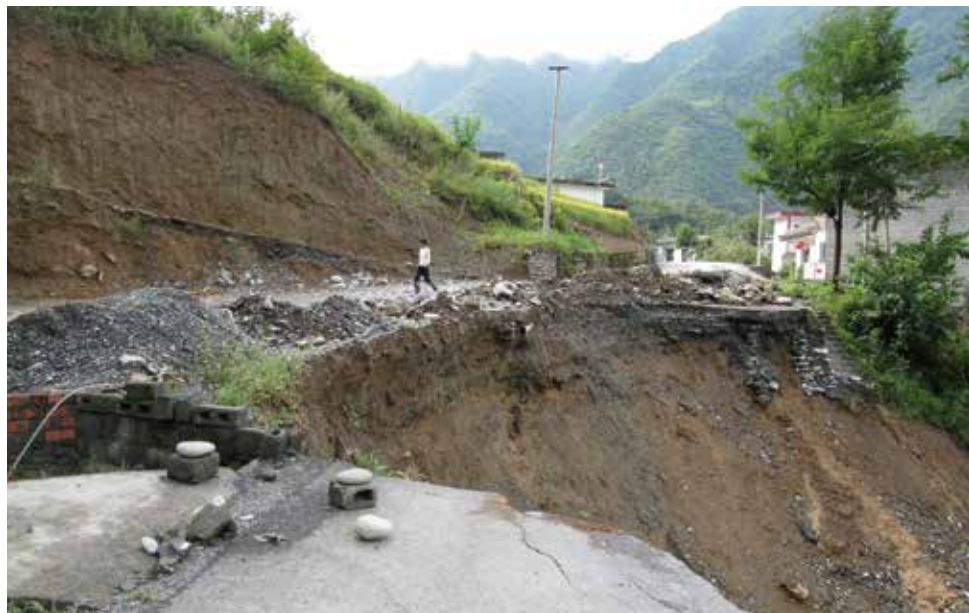
The washed out road from LanGao to Zoujiaping.
