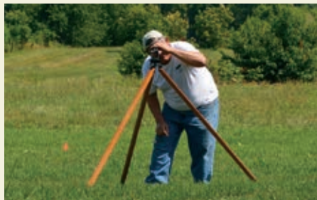
Doug Gillis, using Fred Hebard’s trusty transit, takes a reading on a survey rod held by Jeff Donahue, who is helping do preliminary survey work that will lead to construction of the Field Operations Building at the Price Farm in Meadowview. Photo by Ruth Gregory
